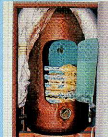
The copper cylinder scales up. This makes it work harder and become less efficient.
