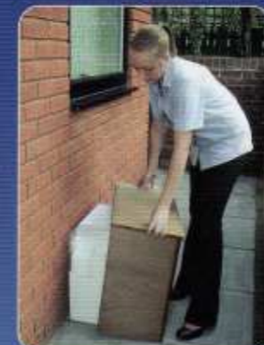
The TwinTec installed in a waterproof housing outside.
